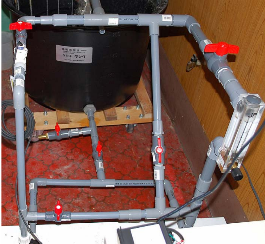
Fig. 3.12: Dual pump and flow meters with PVC plumbing and valves
