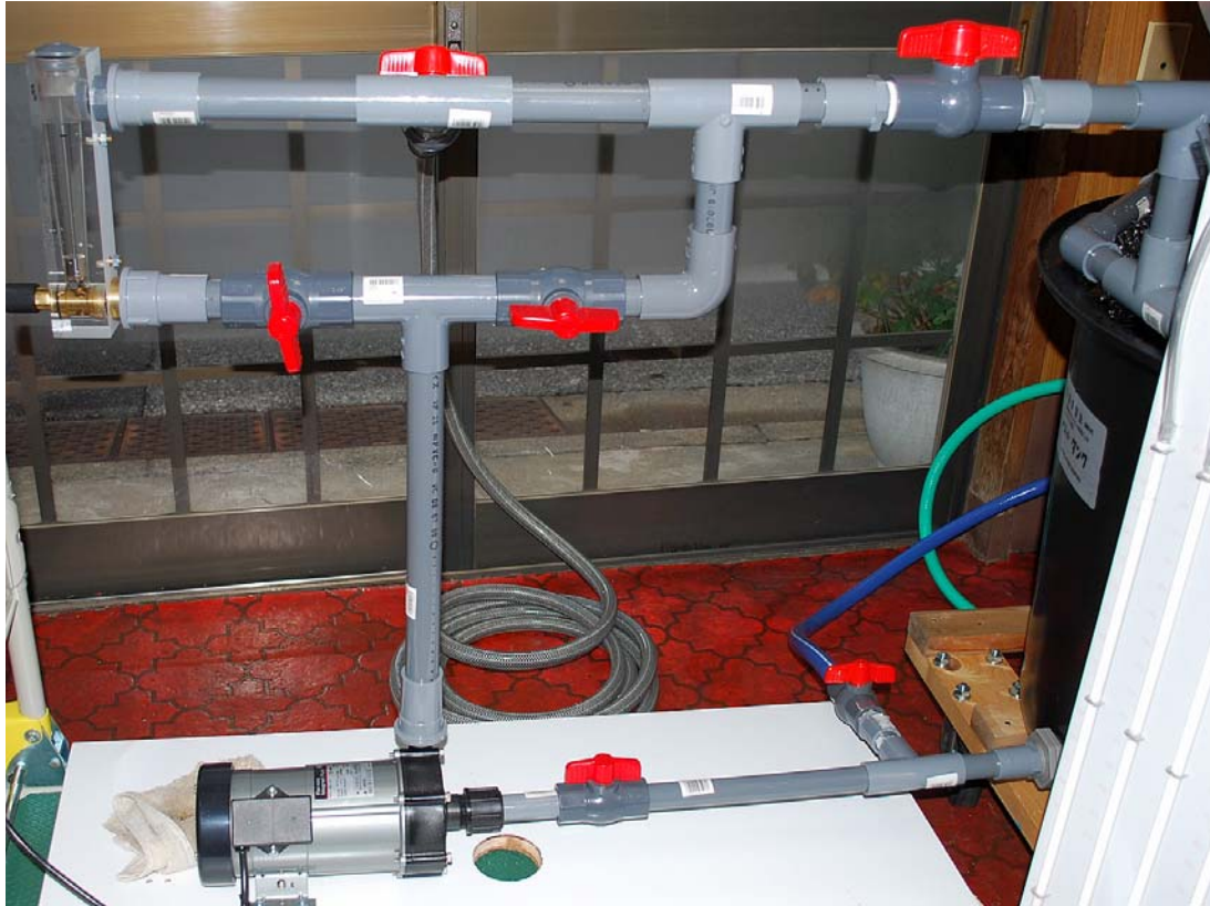
Fig. 3.9: PVC plumbing and valves
