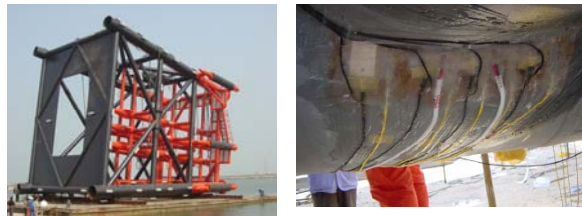
Figure 12 SHM system for CB32A platform
