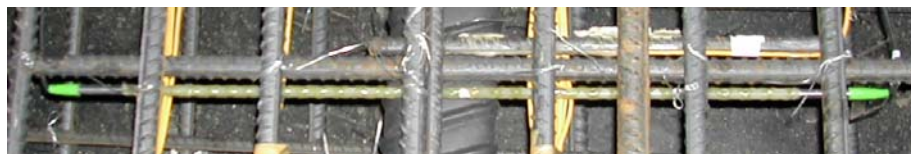
Fig.5: The optical fiber strain sensor installed in the girder.
